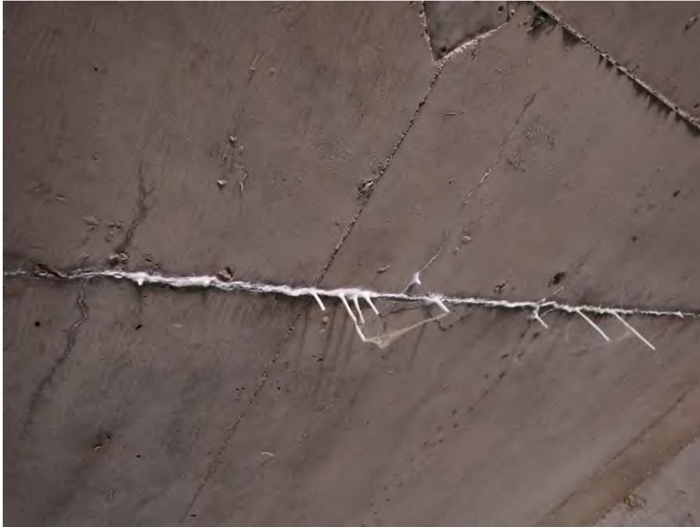
Photo 3: Underside of roof 1/4 way in from the west end, cracking with efflorescence and stalactites full width
