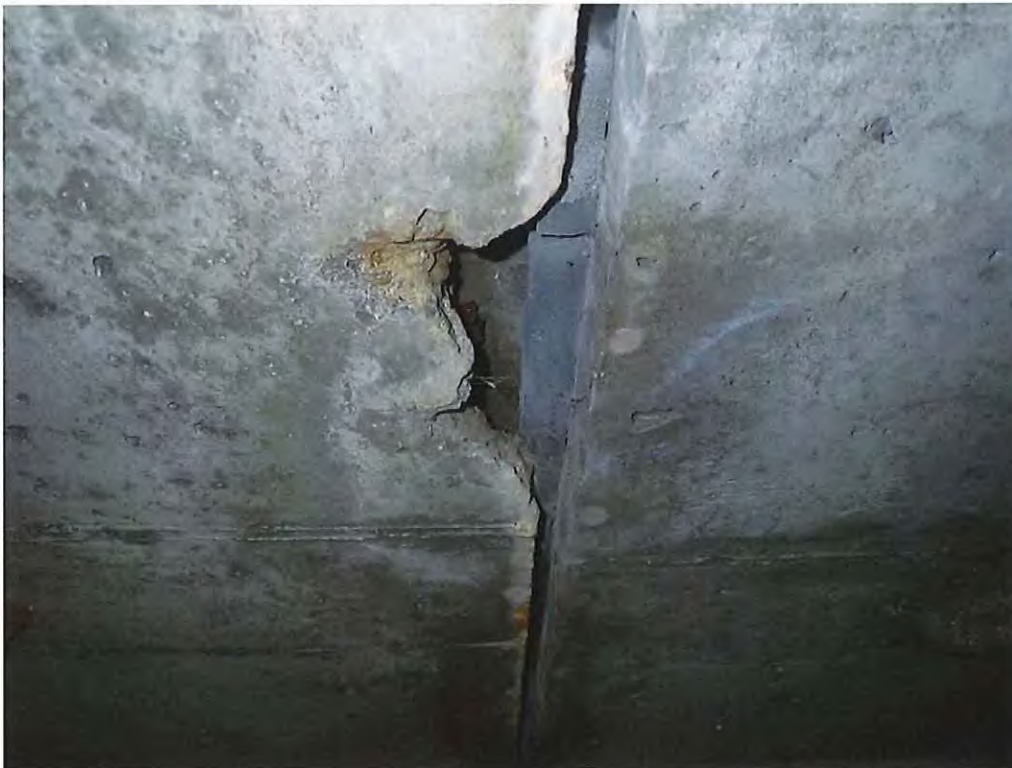
Photo 2: Minor spall in the roof at the south edge of joint #1 in span #1
