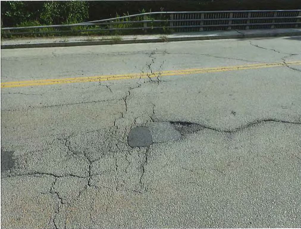
Photo 9: Transverse cracking over the west abutment with bituminous patching and a pothole in the eastbound approach roadway
