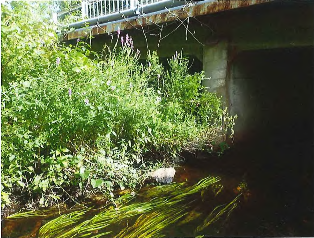
Photo 15: Heavy vegetation and aggradation in front of span #2, upstream end (south end)
