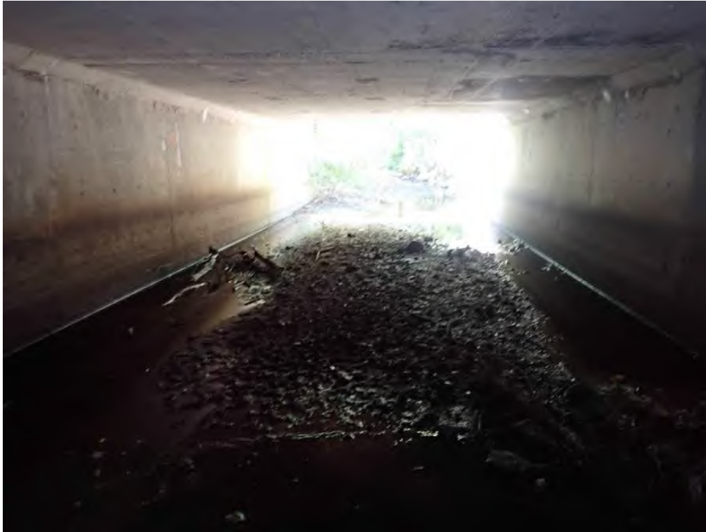
Photo 9: Moderate aggradation at the upstream end in the center of the culvert
