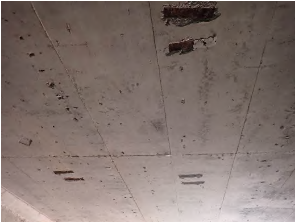
Photo 2: West end of roof, 7', 13' and 18' in, there are three pairs of exposed metal plates, left side, center, and right side of roof
