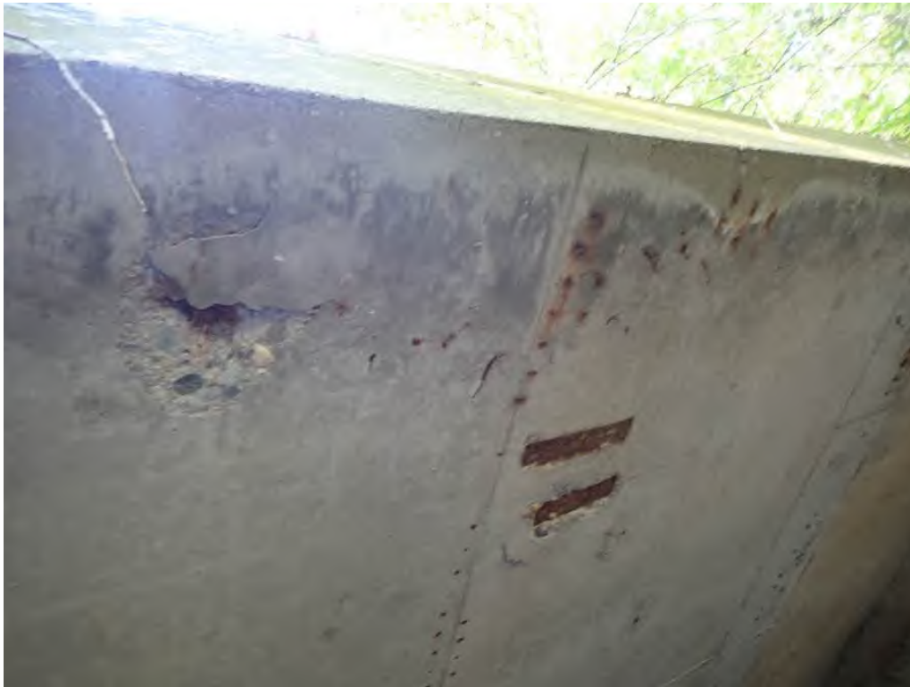
Photo 5: East end of roof, two 2" x 10" exposed metal, one with delamination and minor spall just south of exposed metal at midspan
