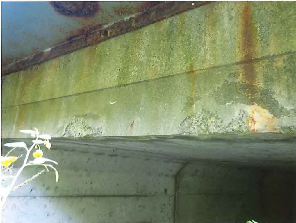
Photo 8: Two minor spalls at the bottom of the south headwall in span #2
