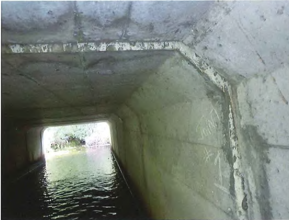
Photo 1: Typical misalignment of roof joints (span #1 at joint #1 shown)
