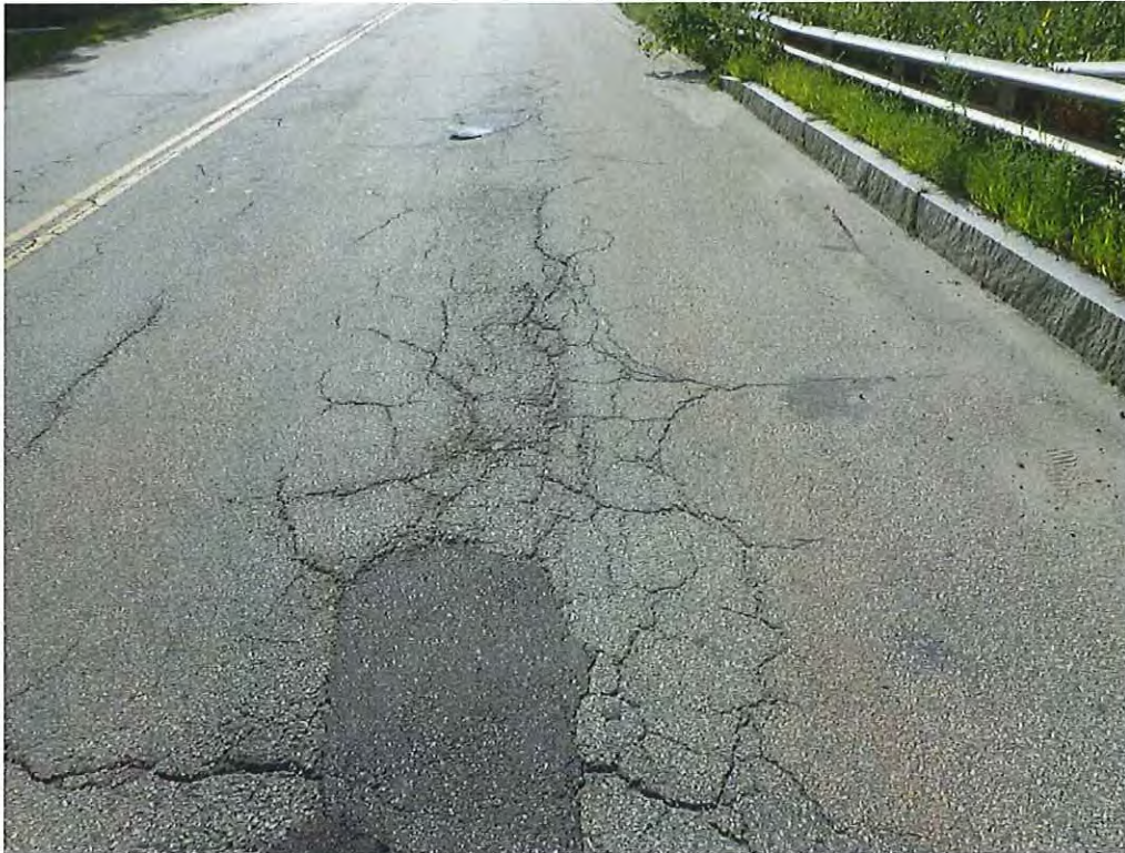
Photo 17: Moderate to heavy map, longitudinal, and transverse cracking in the eastbound roadway at the east approach
