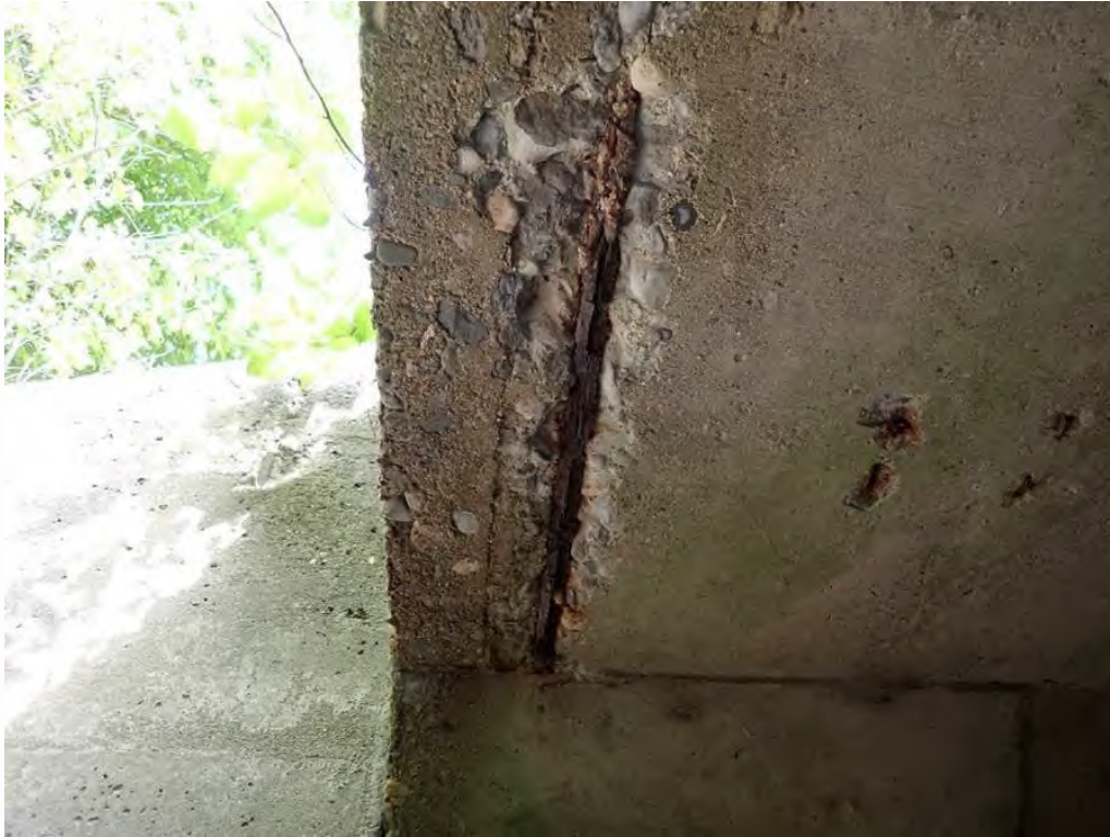
Photo 1: West end of the roof by the north breastwall, spall with exposed rusted rebar with insignificant section loss. Just east, 8 pop-outs with rebar
