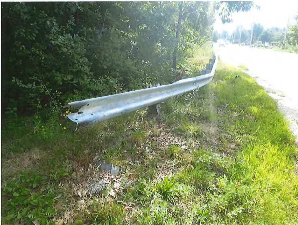
Photo 18: Northwest approach guardrail collision damage has pulled the buried railing out of the ground leaving no end treatment
