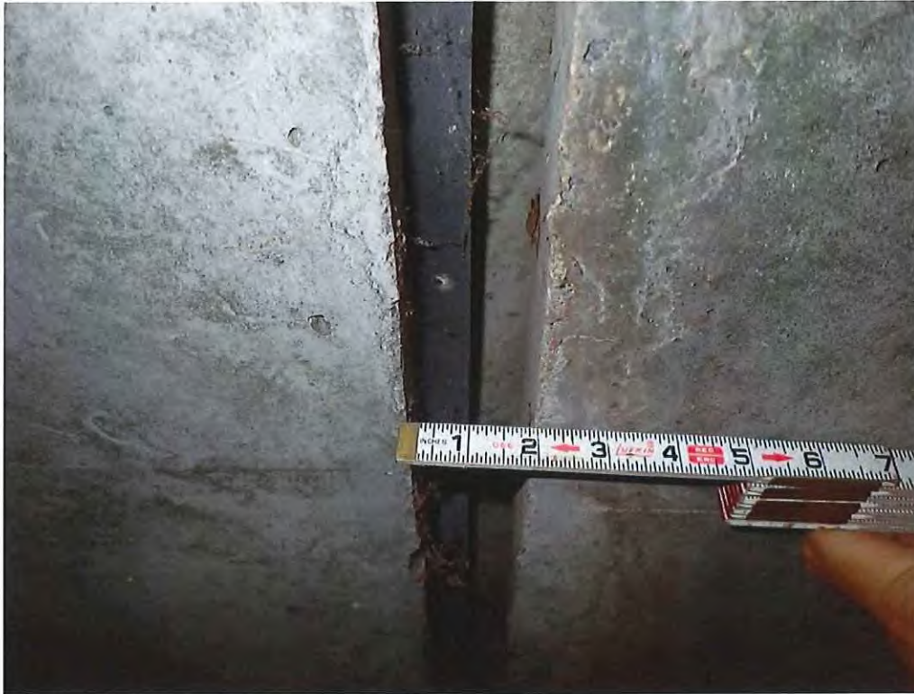
Photo 3: There is a 2" gap between sections in the roof at joint #2 in span #1
