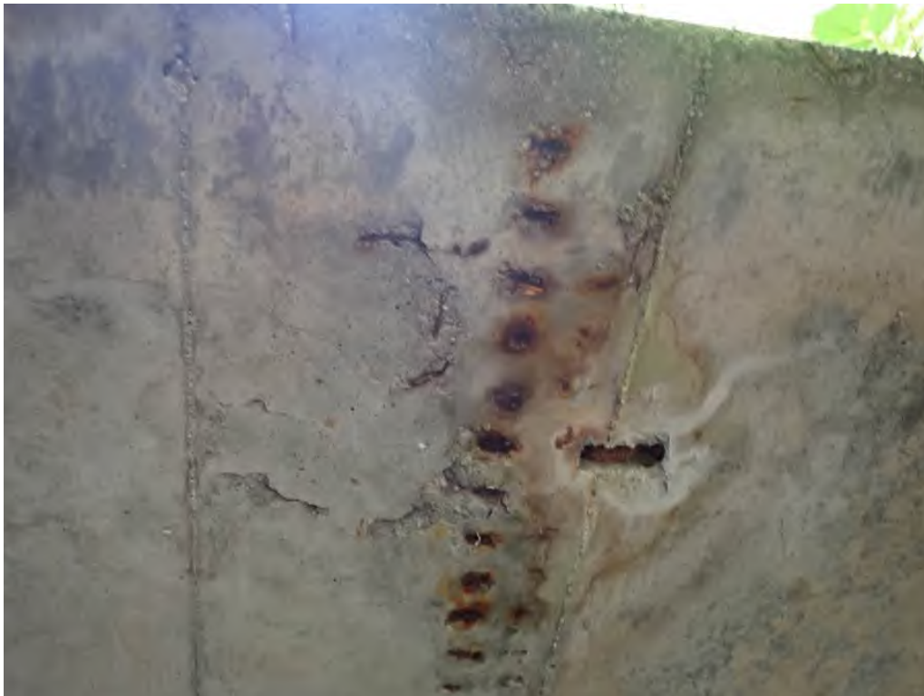
Photo 6: East end of the roof, minor spalling and delamination with exposed metal plates on the north side
