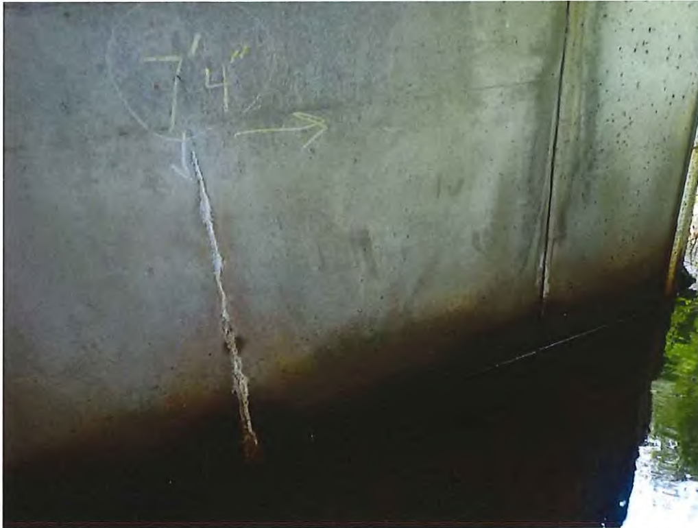
Photo 7: Typical vertical cracks with efflorescence in span #2 at the south end of the west wall
