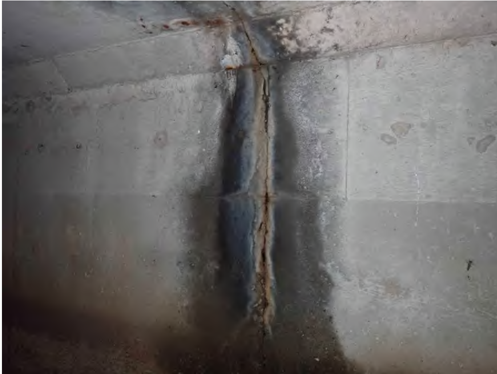
Photo 7: South wall 25' from east end, full height moderate crack, rust, efflorescence, and water staining, same at opposite wall
