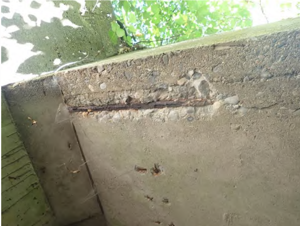
Photo 1: West end of the roof by the north breastwall, spall with exposed rusted rebar with insignificant section loss. Just east, 8 pop-outs with rebar
