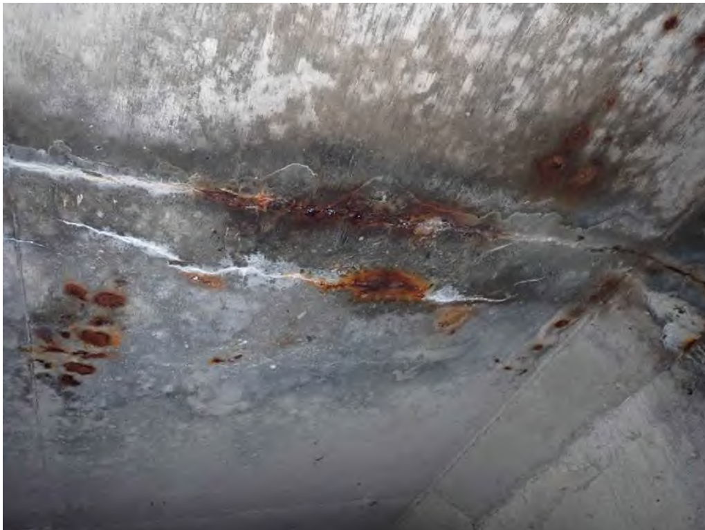
Photo 4: Roof joint 25' from the east end, hairline cracking with efflorescence, rust staining and water staining adjacent to the south wall
