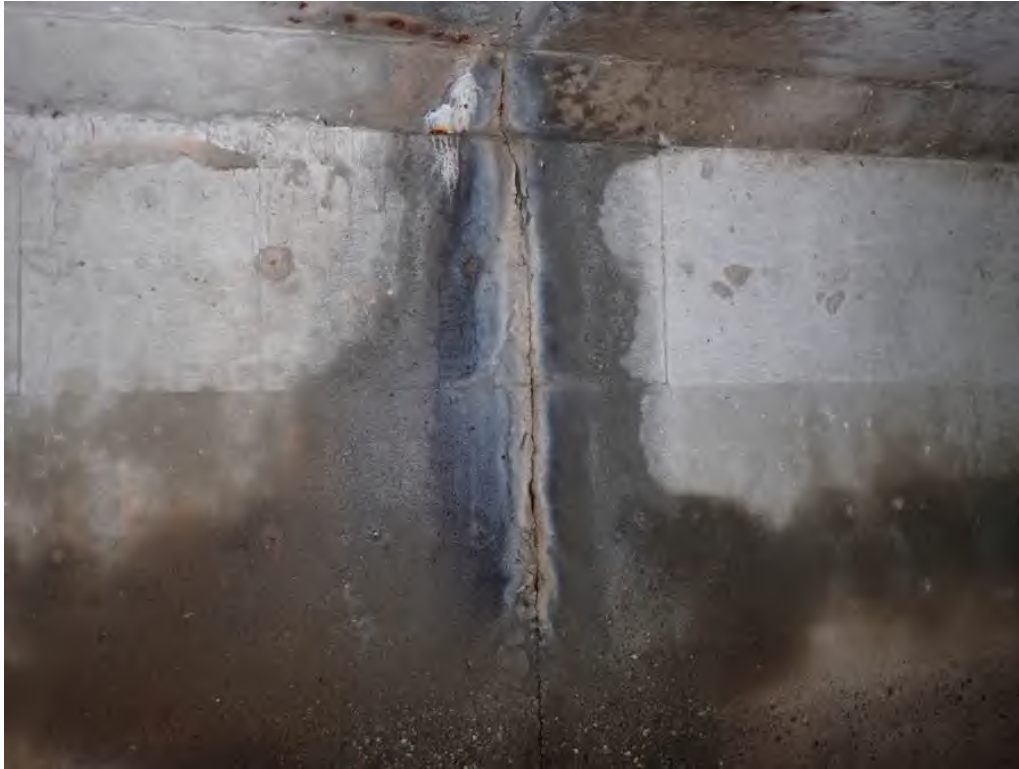
Photo 7: South wall 1/4 way in from east end, full height moderate crack, rust, efflorescence, and water staining, same at opposite wall
