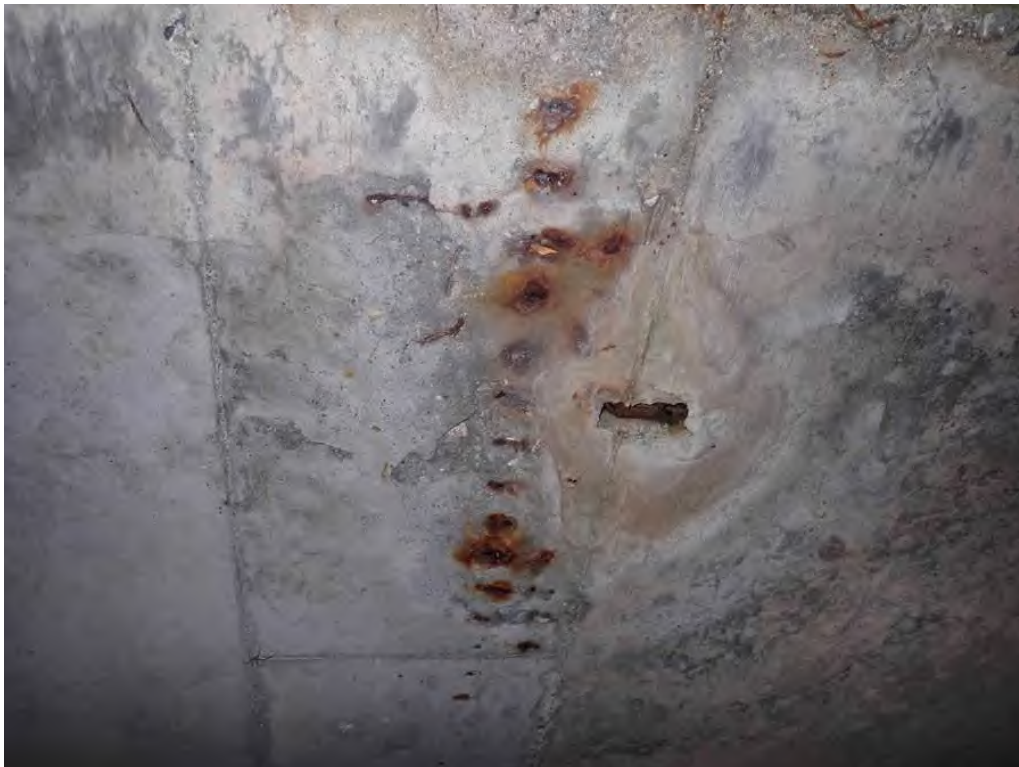
Photo 6: East end of the roof, minor spalling and delamination with exposed metal plates on the north side
