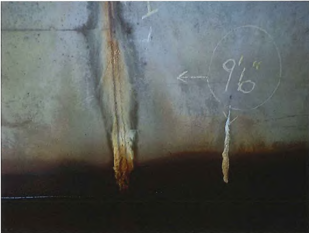
Photo 6: Heavy efflorescence at joint #1 of the west wall in span #1 and typical vertical crack with efflorescence
