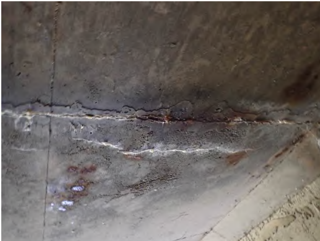
Photo 4: Roof joint 1/4 way in from the east end, hairline cracking with efflorescence, rust staining and water staining at south wall
