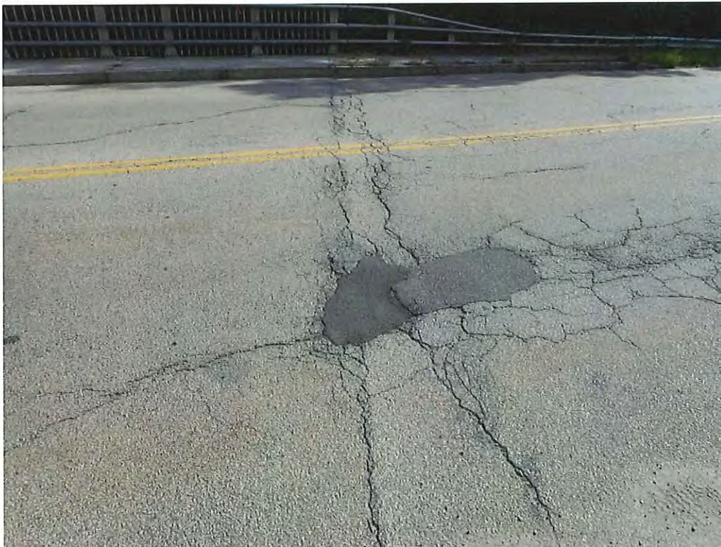
Photo 10: Moderate cracking over the east abutment with bituminous patching in the eastbound roadway extending into the east approach
