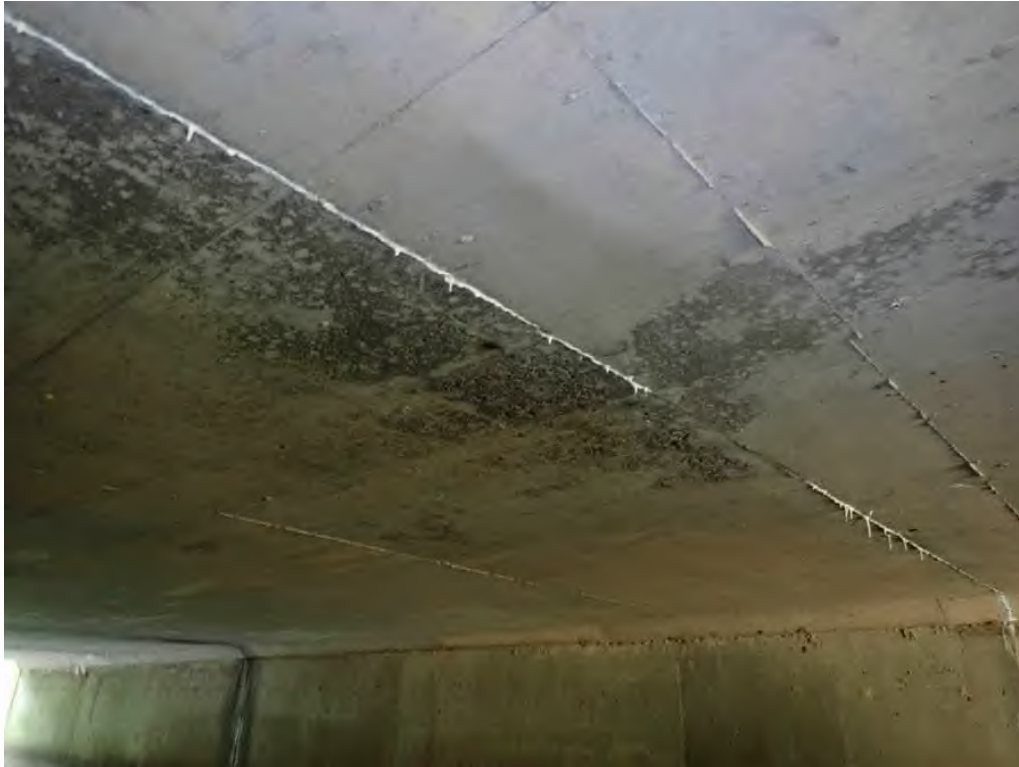
Photo 3: Underside of roof 25' from the west end, cracking with efflorescence and stalactites full width
