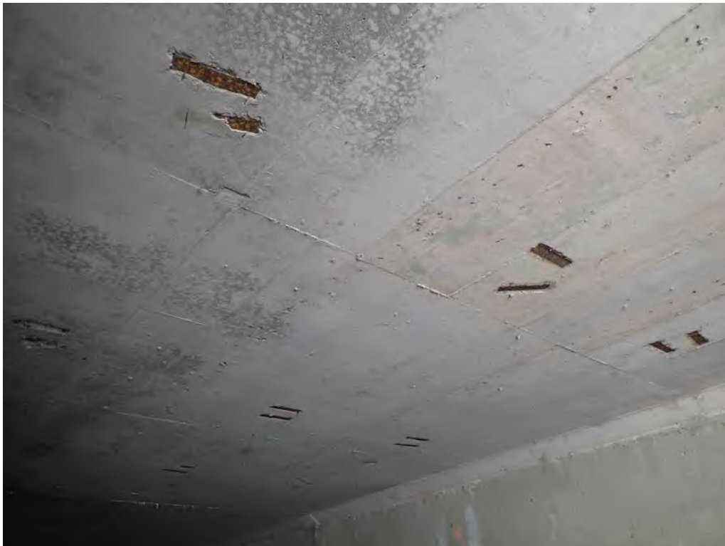
Photo 2: West end of roof, 7', 13' and 18' in, there are three pairs of exposed metal plates, left side, center, and right side of roof
