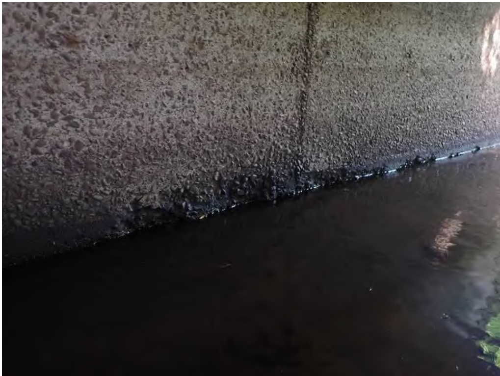
Photo 8: Ratholing at the waterline along the north wall by the east end
