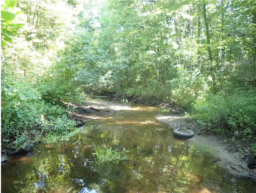
Photo 11: Downstream (east end) of culvert, aggradation, debris and vegetation along banks
