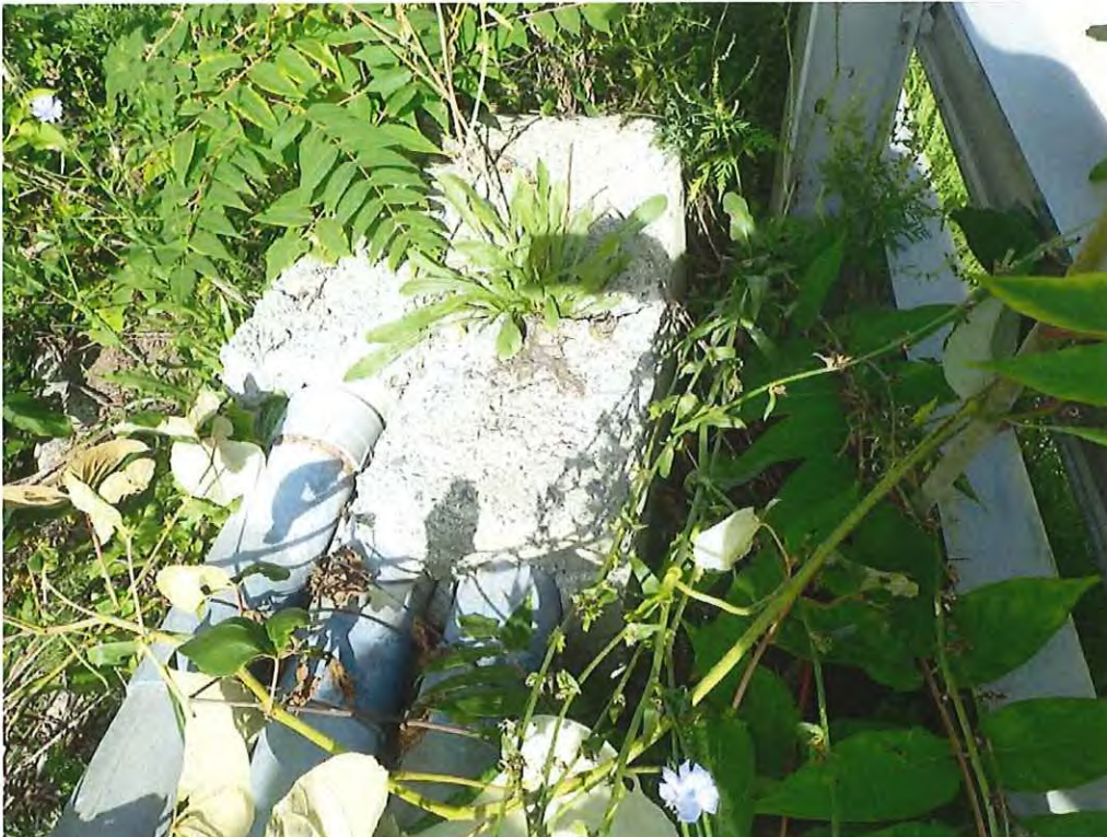
Photo 12: Cracking and scaling of the concrete encasement at the southwest end of utilities
