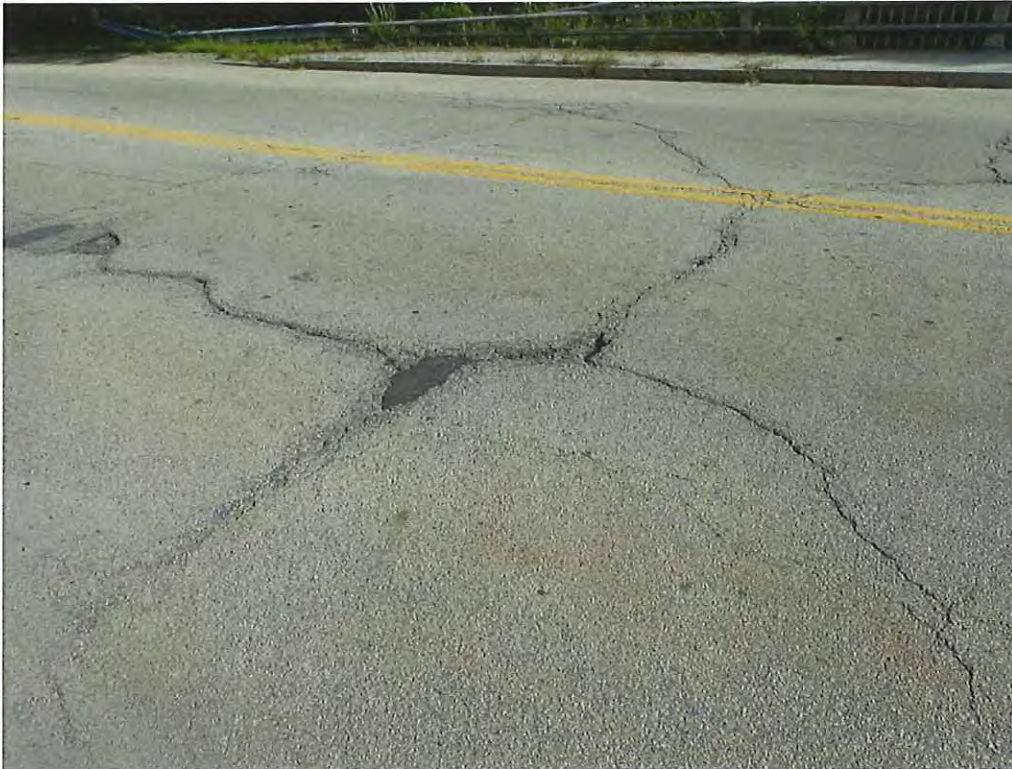
Photo 11: Typical moderate cracking with bituminous breaking up in the wearing surface, note pothole near midspan of eastbound travel lane
