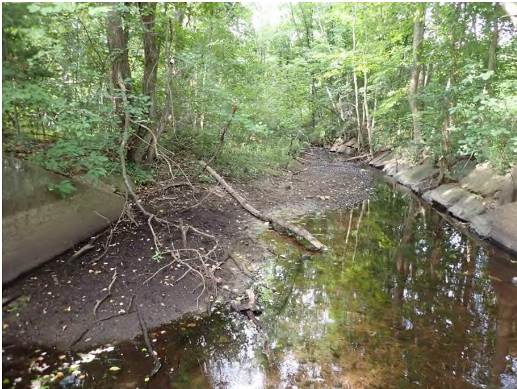
Photo 10: Aggradation upstream (west end) of river restricting channel
