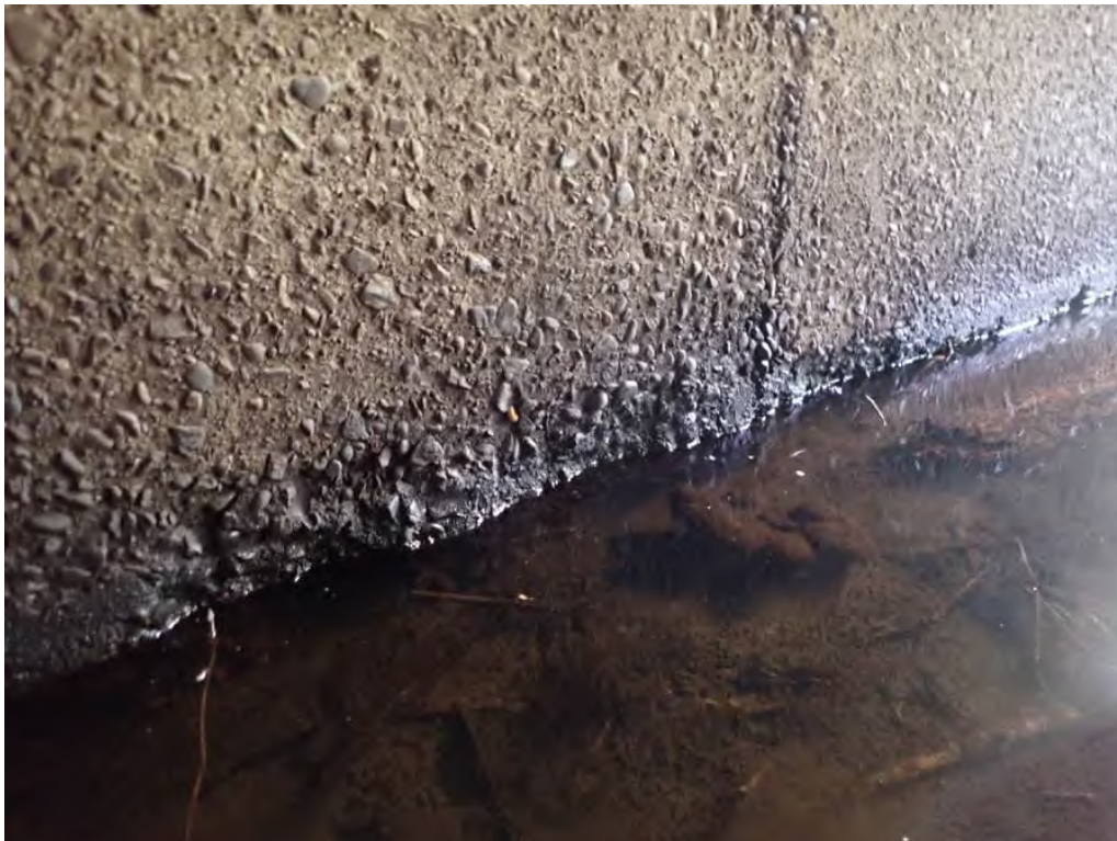
Photo 8: Ratholing at the waterline along the north wall by the east end
