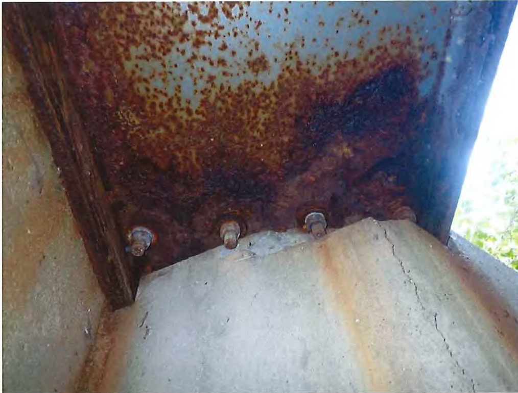
Photo 13: Typical heavy rusting with lamination at the edges of the steel support (below utilities)
