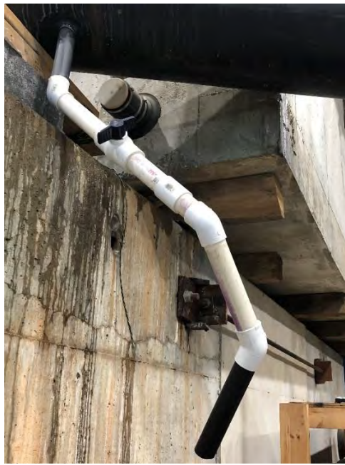
Figure 8 Photograph of Background Sampling Port
