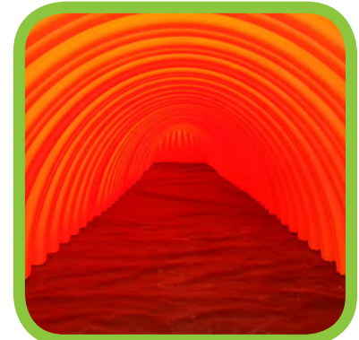
Looking down the Isolator Row from the manhole opening, woven geotextile is shown between the chamber and stone base.
