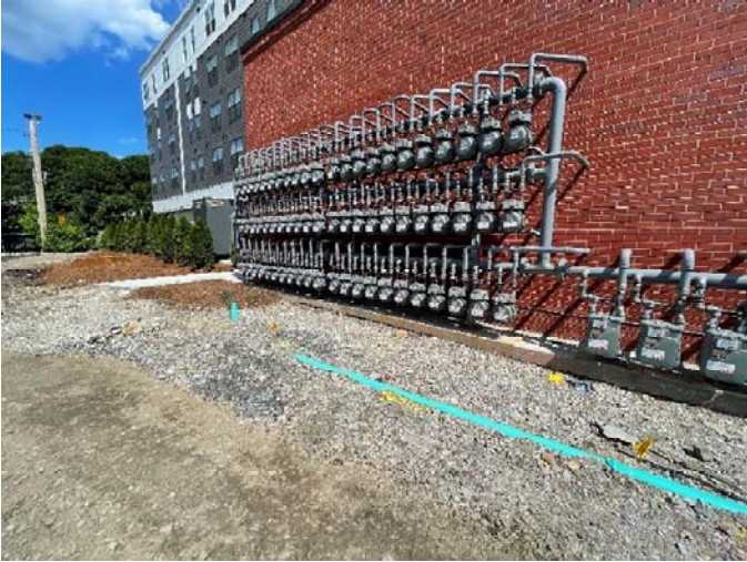
View of gas meters
