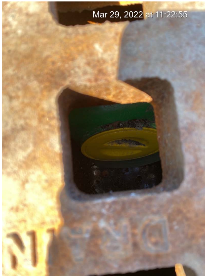
Photo 2 – Installed Oil Snout/Hood #1 Retrofit
