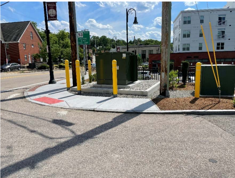
Generator surrounded by bollards near ADA ramp on sidewalk facing West.
