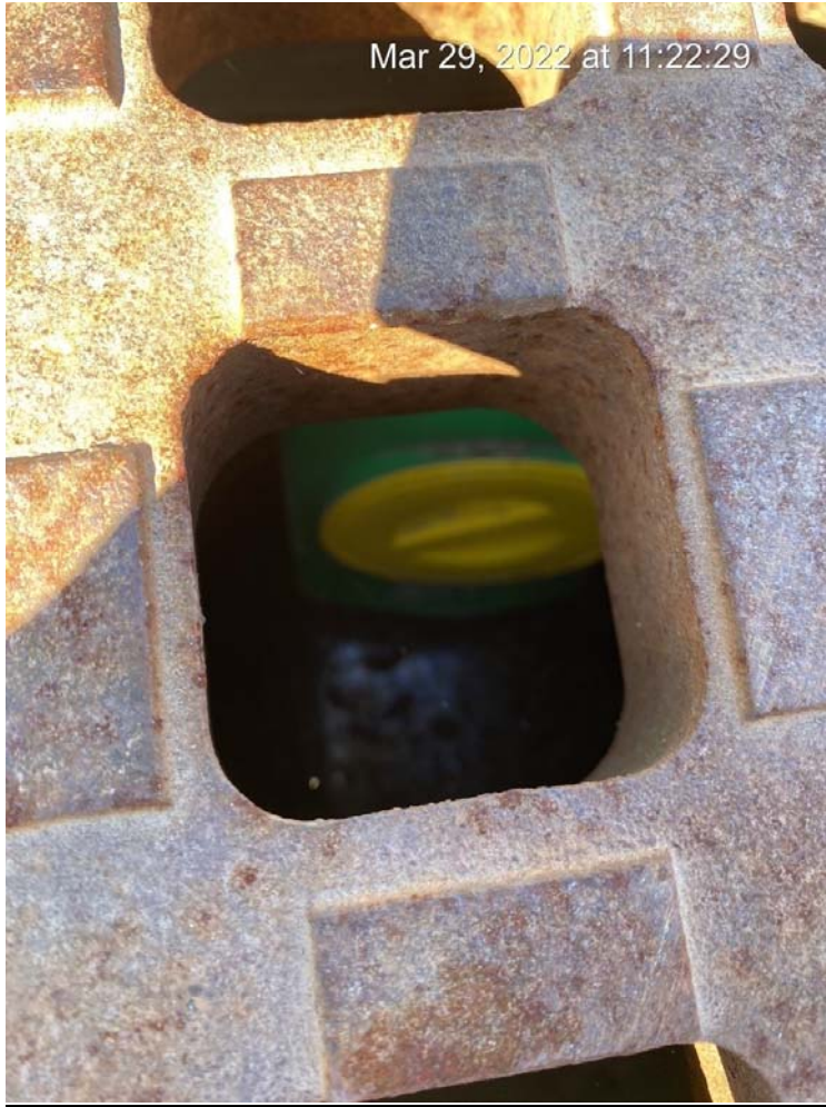
Photo 3 – Installed Oil Snout/Hood #2 Retrofit
