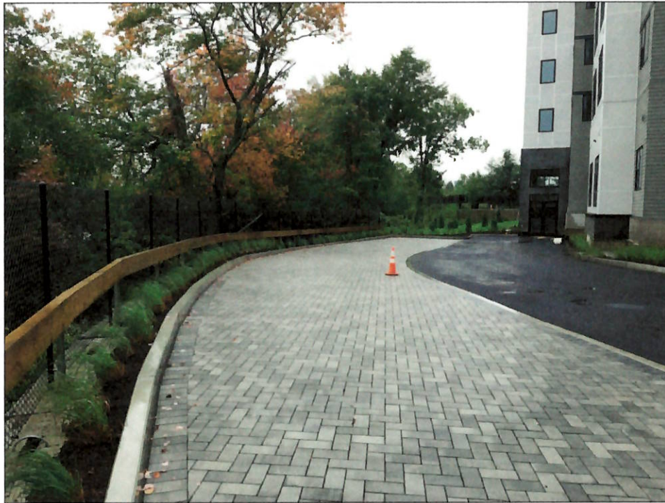
VIEW OF LOOKING SOUTHEAST OF POROUS PAVER PARKING AREA TOWARD POOL AND AMENITIES AREA
