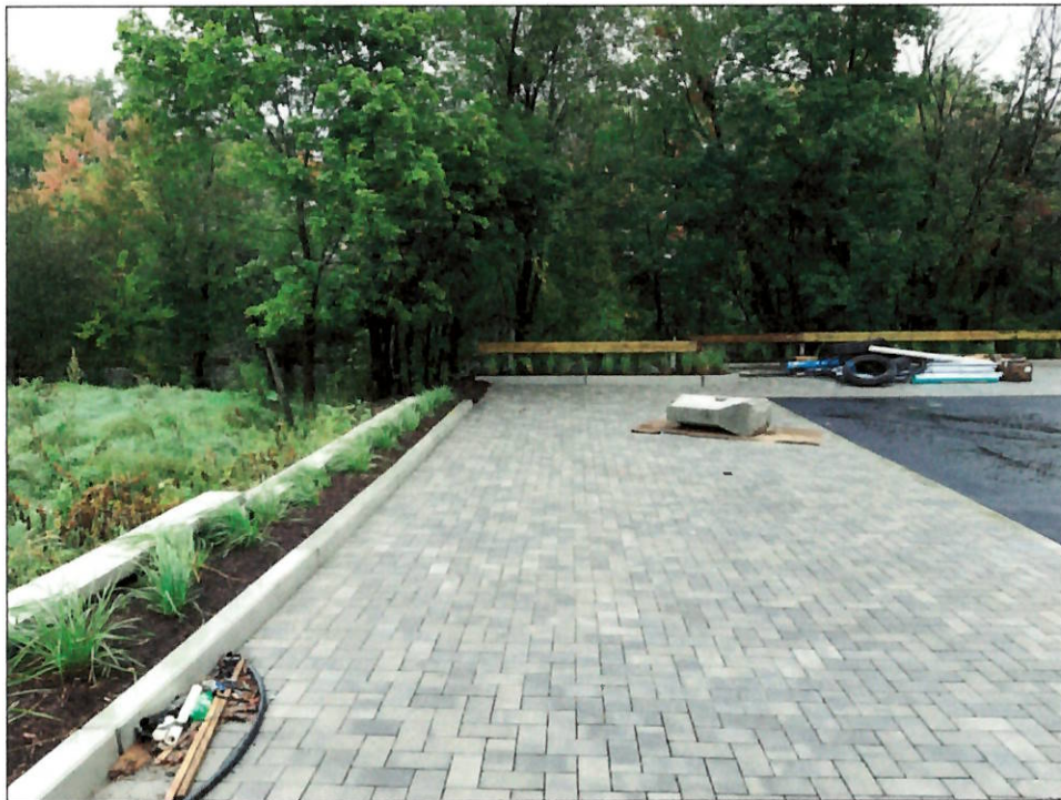
VIEW LOOKING EAST OF POROUS PAVER PARKING AREA AT NORTHEAST CORNER OF SITE
