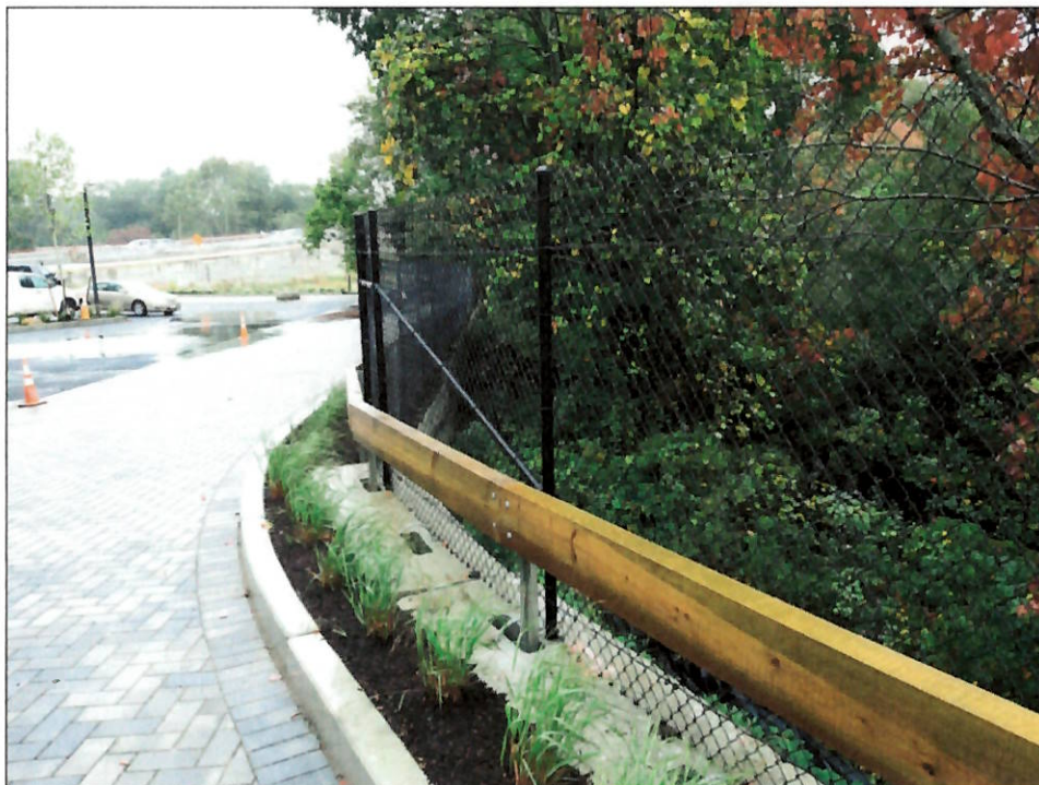
VIEW OF LOOKING NORTHWEST OF POROUS PAVER PARKING AREA AND RETAINING WALL AT EAST SIDE OF SITE
