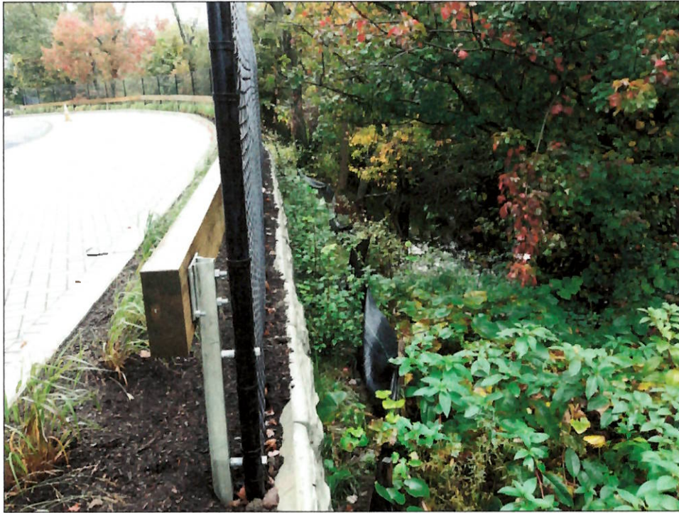
VIEW LOOKING NORTH OF FENCE AND RETAINING WALL ALONG EAST SIDE OF SITE NEAR SOUTHEAST CORNER OF POROUS PAVER PARKING AREA
