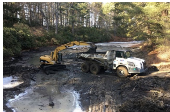
Conventional dry dredging allows for direct loading of excavated sediments from dewatering locations or stockpiles into a hauler.
