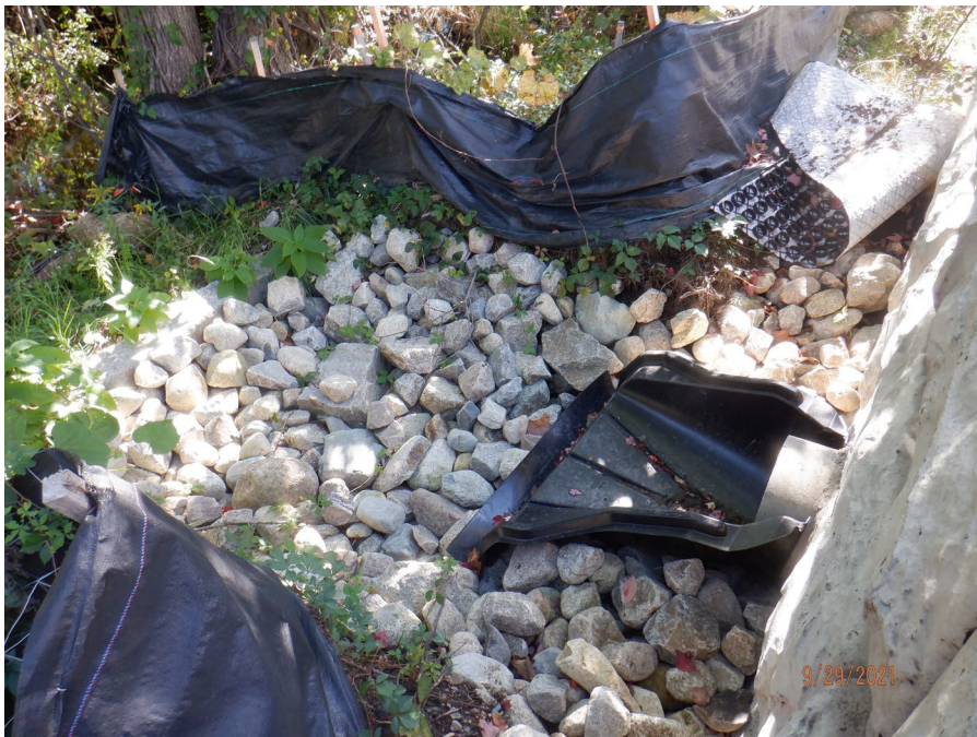
Photograph 12: Stormwater outlet #2, erosion control barrier, and construction debris.
