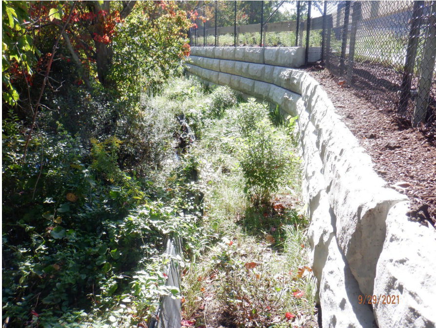
Photograph 1: Typical vegetation between the retaining wall and erosion control barrier, includes planted sweet pepperbush and a mix of herbaceous vegetation.
