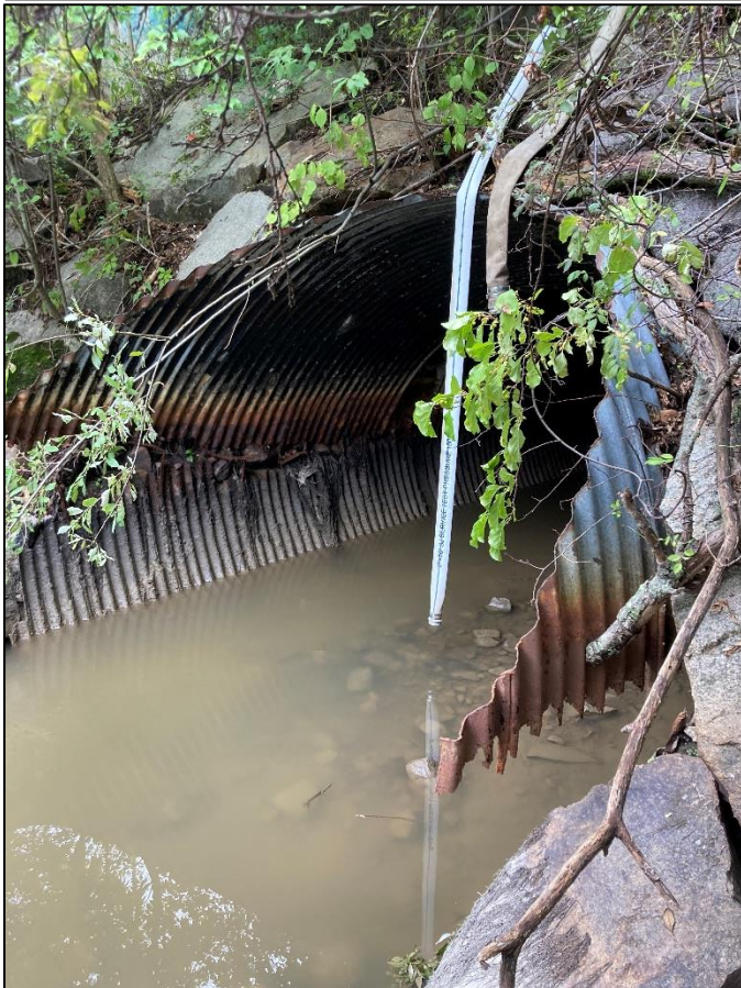
Photo 2. Culvert outlet, before repair 9/7/2022
