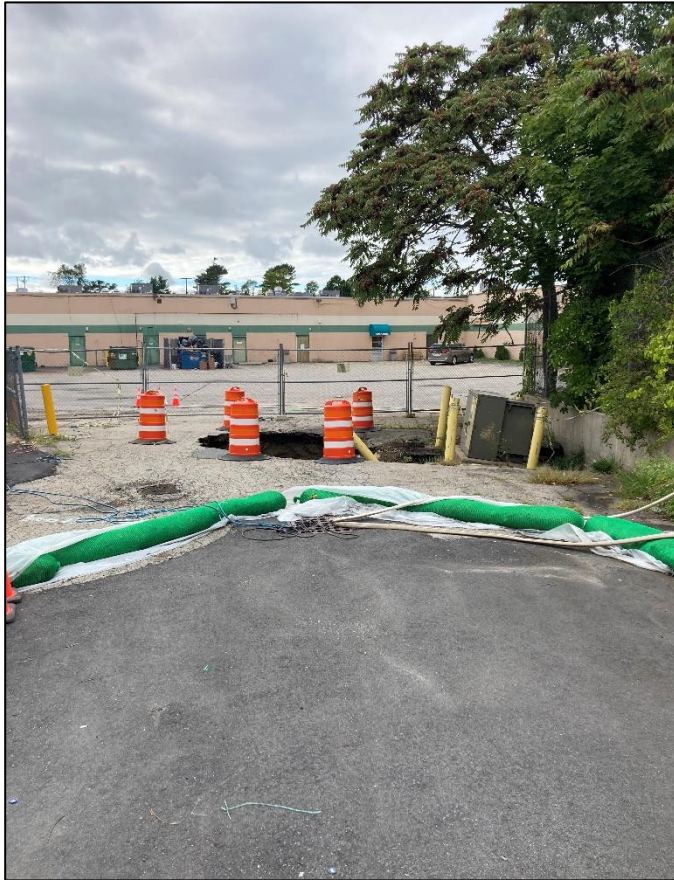
Photo 1. Sinkhole in parking lot resulting from culvert collapse 9/7/2022
