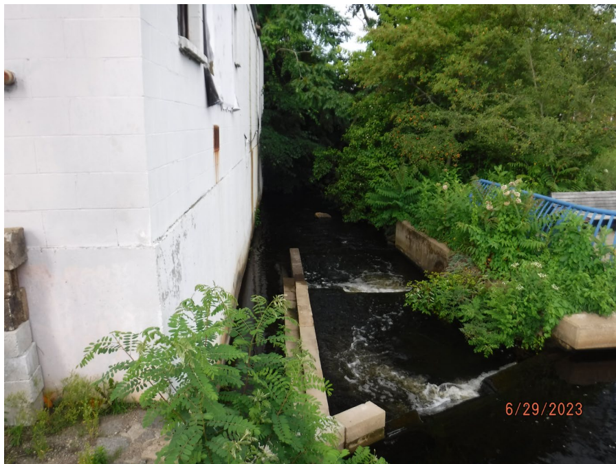
Photograph 20: View of the existing edge of the Venetian Building along the Herring Brook, facing north toward Broad Street.
