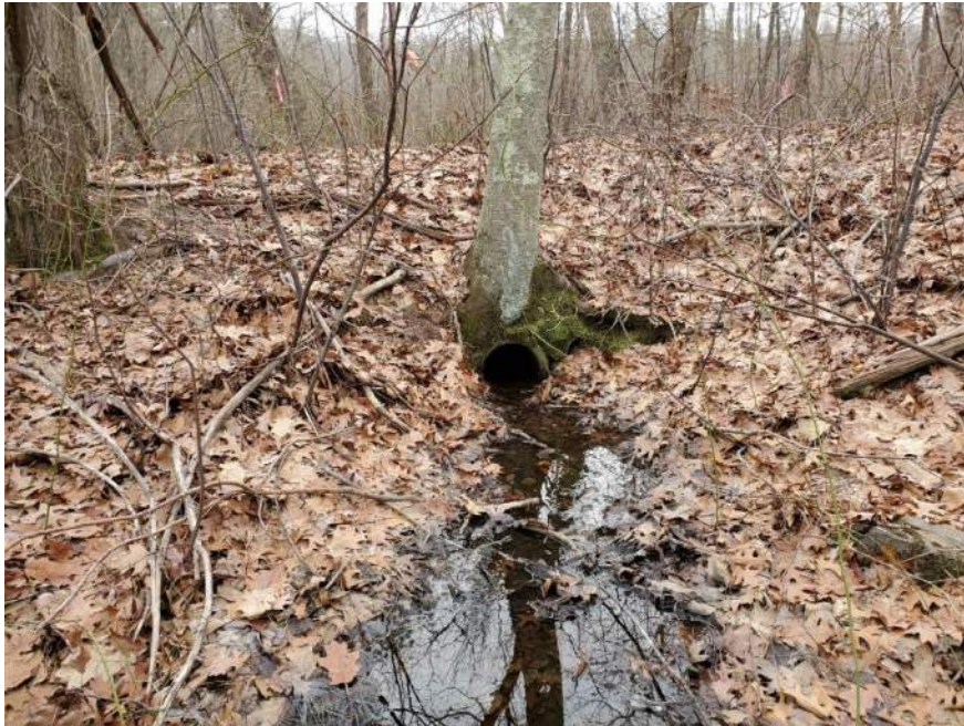
Photo 9: View of culvert to be removed and restored. The culvert is located under the existing access road, at the northern extent of the proposed wetland replication area.
