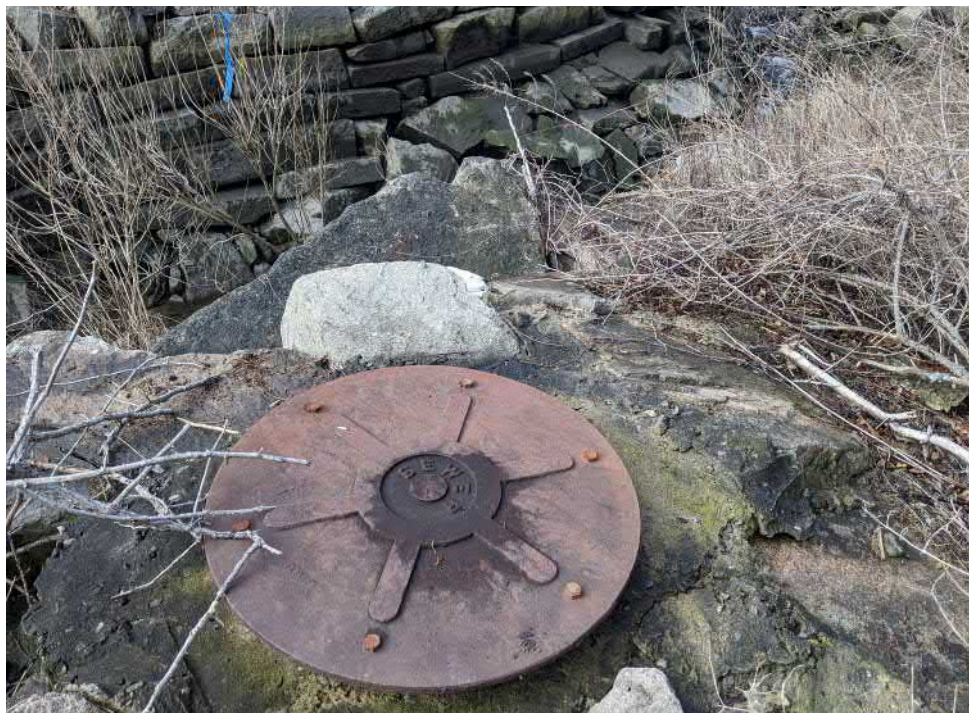
View of a sewer manhole adjacent to the stream shown in Photo 6—facing west.
