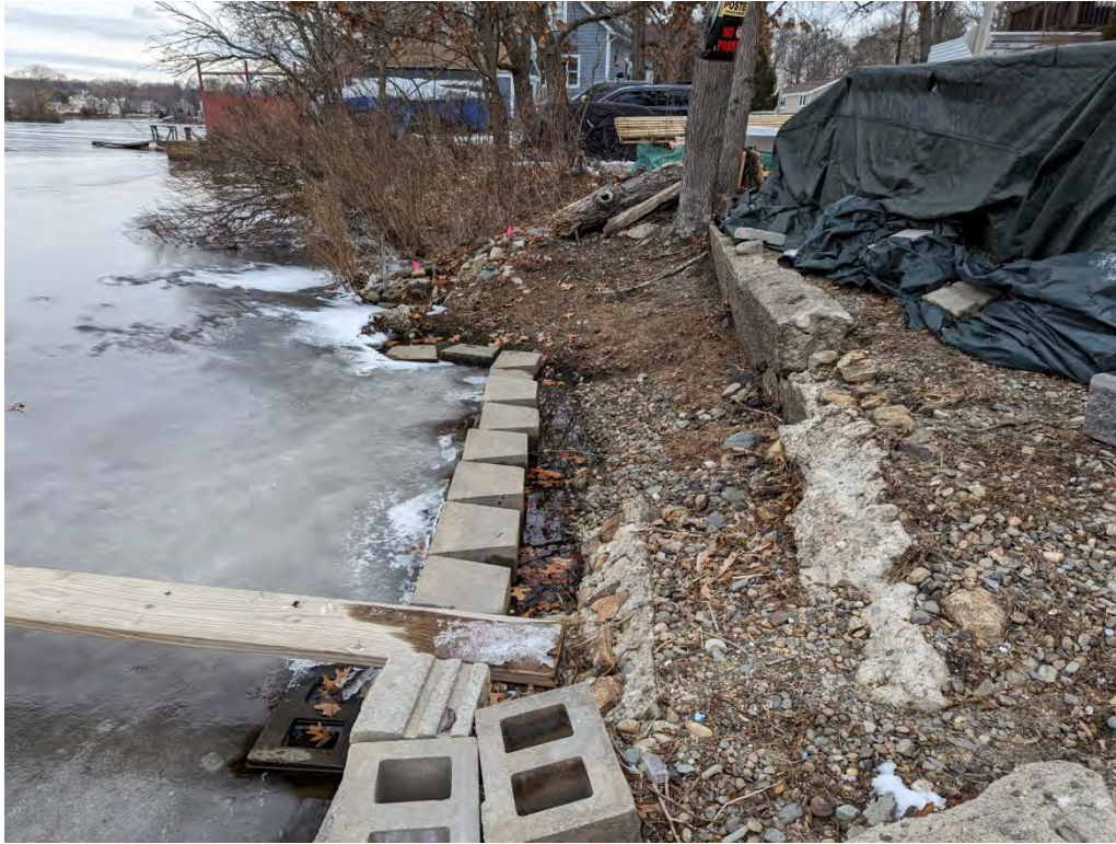
Northern view of the wall base which impacts 22 square feet to Land Under Waterbodies and Waterways and 37 linear feet of Bank
